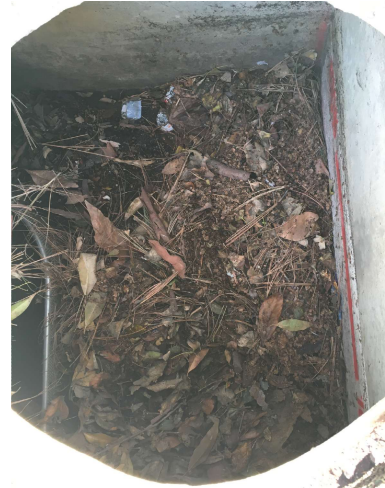
Figure 5.2: Accumulated Trash and Debris in CPS Unit
