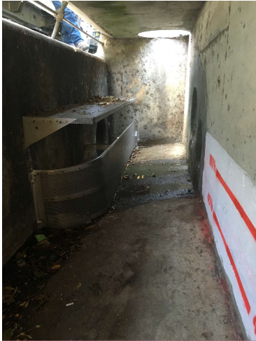
Figure 5.1: Installed CPS Unit
