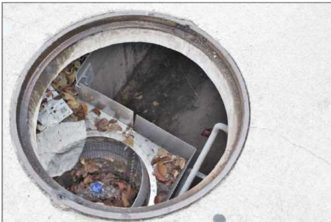
Figure 25 - View 2 of Catch Basin Bottom with Bio Clean® Curb Inlet Filter Installed
