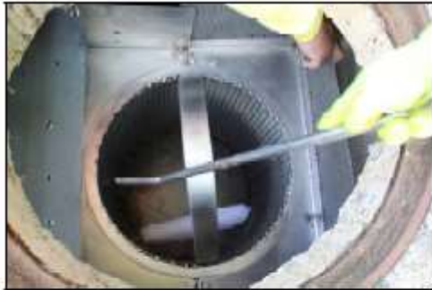
Figure 19 - Curb Inlet Filter Basket Installed In Tray System.
