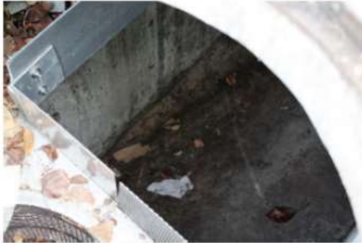
Figure 26 - View 3 of Catch Basin Bottom with Bio Clean® Curb Inlet Filter Installed
