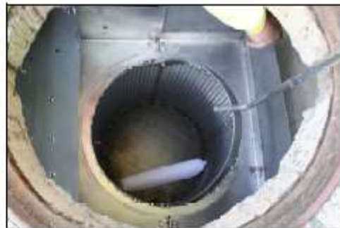
Figure 20 - Curb Inlet Filter Basket Installed In Tray System.
