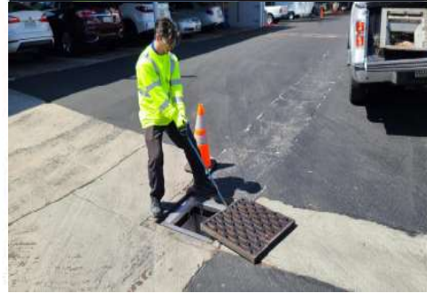
Figure 14 - Grate Inlet Filter (no access window) Installed After Maintenance.
