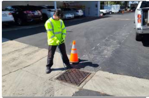
Figure 15 - Grate Inlet Filter (no access window) Installed After Maintenance.
