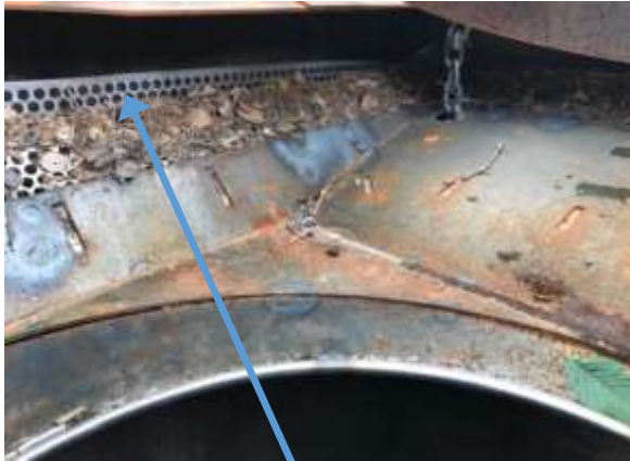
Image 6 - DIF with progressive overflow trash screen
