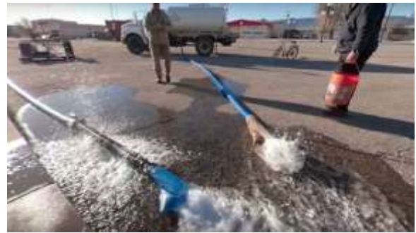
Image 18 - Combined test water sources output. Adjustable hydrant meter max capacity 350 GPM Pressurized water truck max capacity 150 gpm
