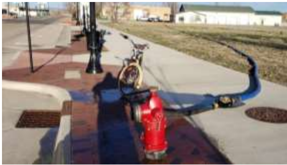
Image 17 - Adjustable hydrant meter water source - up to 350 gpm
