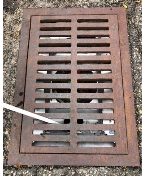
Image 15 – Opening pivot sample port through grate hole with 1" PVC pipe
