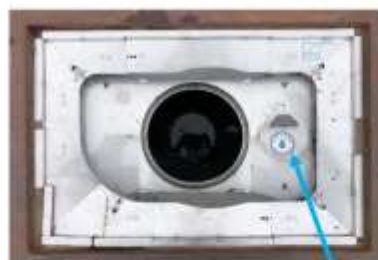
Fig. 4 - 5" diameter pivoting sample port on filter hanger in closed
