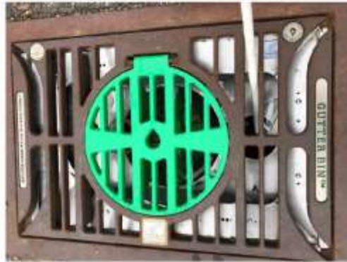
Image 9 – Sample port being pivoted with grate in place to view bottom of catch basin
