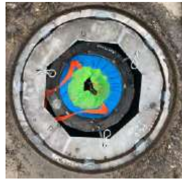
Image 24 – Device in round catch basin. Vector control achieved around filter hanger as one can see the bottom of the catch basin from above.
