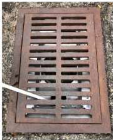
Image 3 - opening sample port through grate hole with 1" PVC pipe
