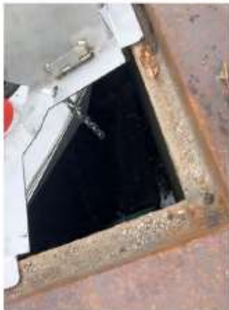
Image 11 – View of the catch basin sump through the hinged sample port located on the frame.
