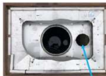
Fig. 5 - 5" diameter pivoting sample port on filter hanger in open
