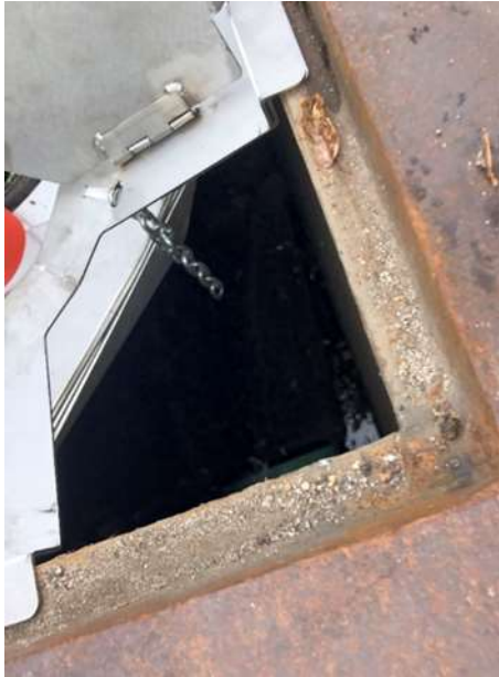
Image 14 – Open hinged sample port located on UGF to view catch basin
