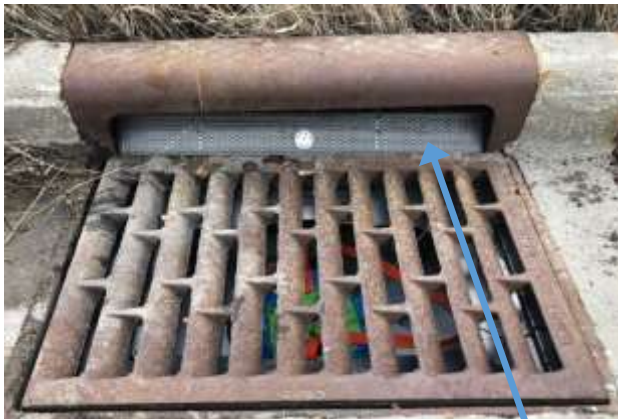
Image 4 – Installed DIF-C below the existing storm grate cover and an inlet screen in curb inlet opening
