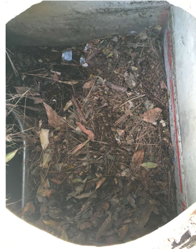
Figure 5.2: Accumulated Trash and Debris in CPS Unit
