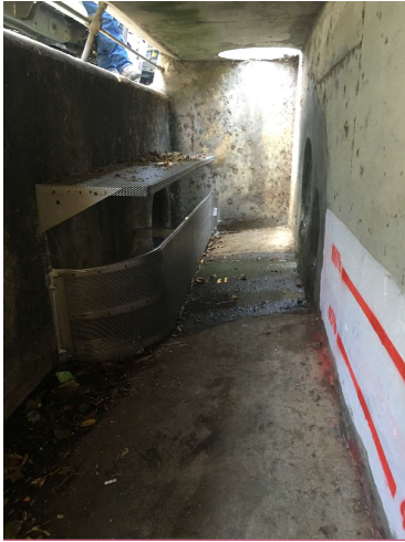
Figure 5.1: Installed CPS Unit
