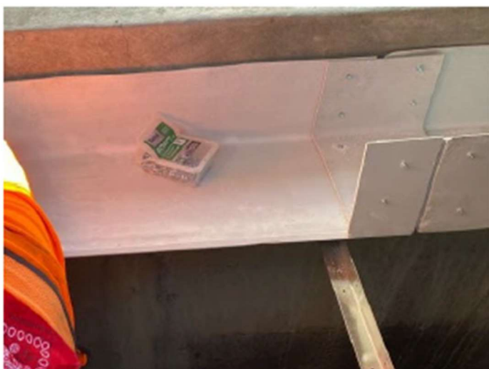
Example installation where a 2' trough section has a section cutout that matches the bridging struts.
