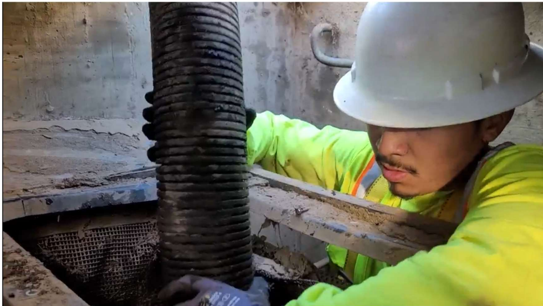
Figure 31 Example of a contractor maintaining the Enviropod® LittaTrap™ High Capacity from within the catch basin having entered via the manway.
