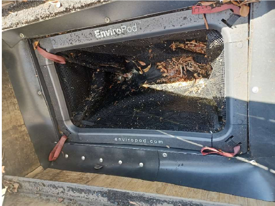
Figure 37 EnviroPod® LittaTrap™ FC LT9060 with HVPS installed in a grated inlet (Configuration 1)
