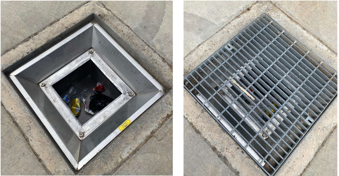
Figure 28 Example of the stainless-steel basket installed in a grate inlet catch basin (Configuration 1)
