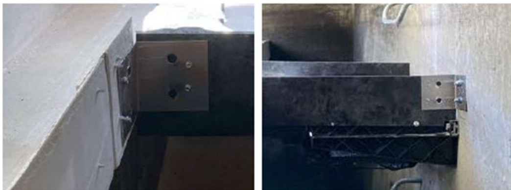
4x4 bracket installation attaching the headwall to the trough (left) and the concrete cb wall (right).
